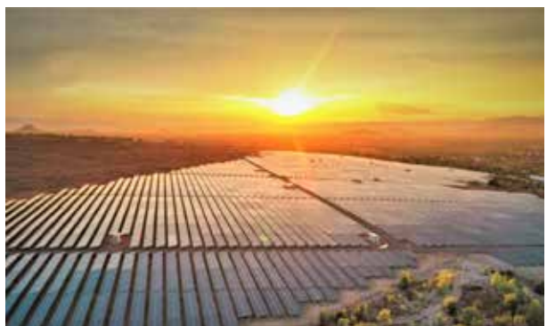
Song Luy 1 Solar Power Plant (47MWp)
