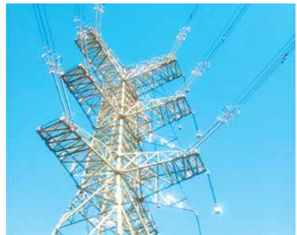
500kV Duyen Hai Transmission line Tower - EPC Package Duyen Hai 2 TPP
