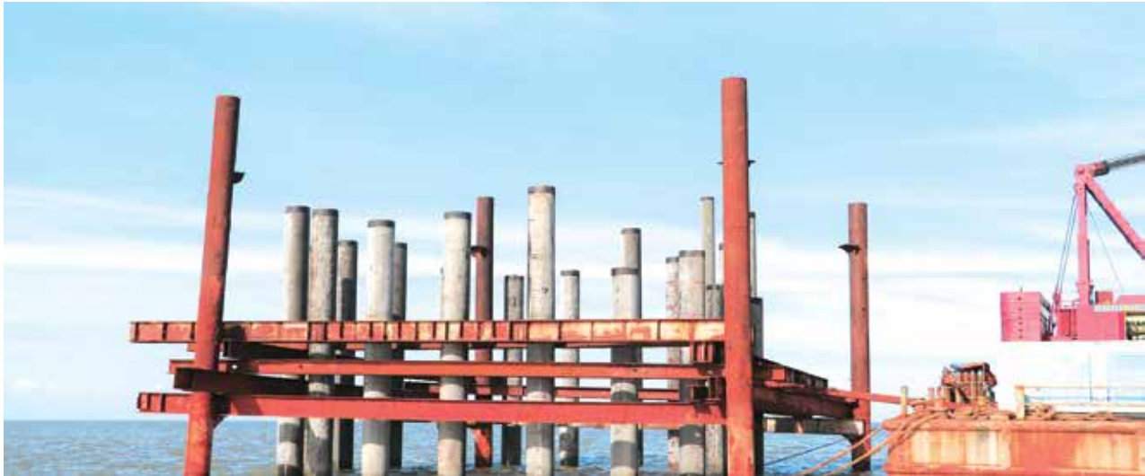
Tan Thuan Wind Power Plant Project - EPC
