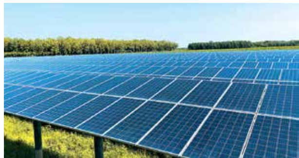
Dau Tieng 3 Extension Solar Power Plant (108MWp)
