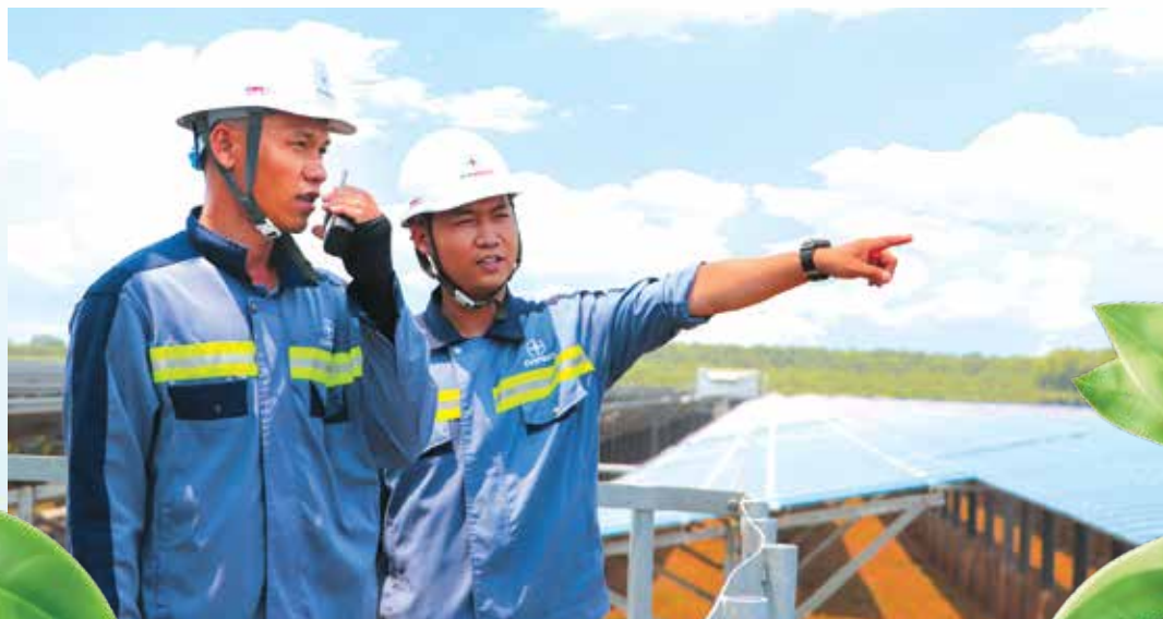
Dau Tieng 3 Extension Solar Power Plant (108MWp)
